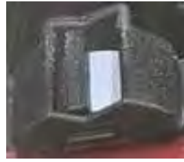
White field: Direction of rotation incorrect: Flow in the temperature control circuit too low
